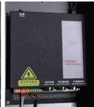
SERVO CONTROL BOX
